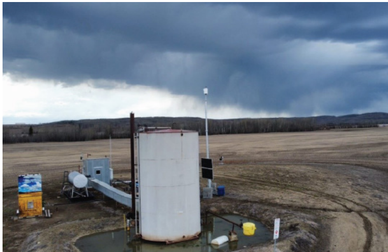
Figure 12: ETC Vent Site with different emission points and On-Site Combustor
