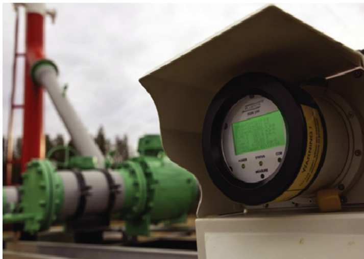
Figure 8: Flare System Bypass Flanges and Fluenta Flow Indicator
