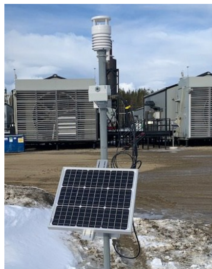
Figure 32: Luxmux Smartpole setup at the ETC Gas Plant Testing Site
