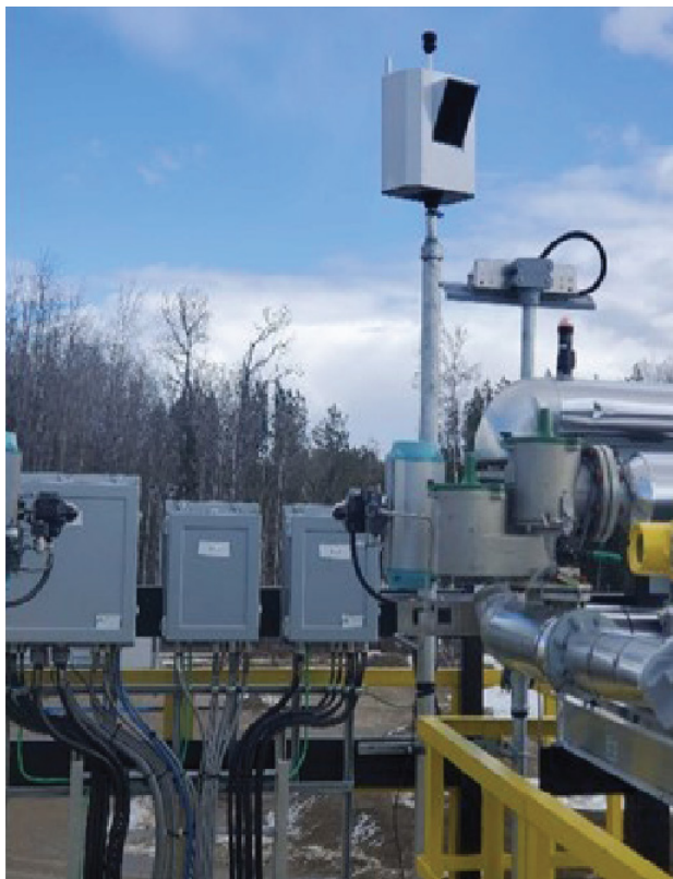
Figure 25: Kuva Camera East Installation
