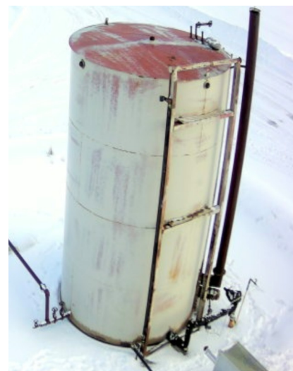
Figure 30: Camera view of ETC 13-35 Well Site
