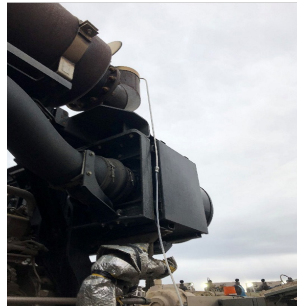
Figure 34: Exhaust sample line connected to a Tier 4 engine
