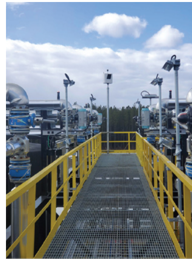
Figure 27: Kuva Camera West Installation
