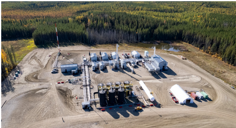
Figure 6: Aerial image of Tourmaline’s West Wolf Lake Gas Plant
