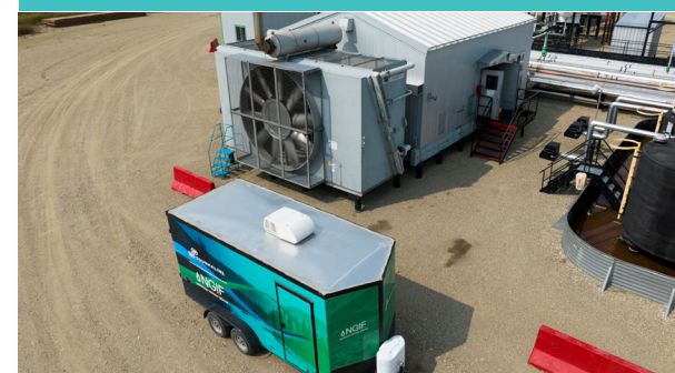
The Continuous Emissions Monitoring System (CEMS)
